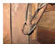
Poor wiring connections without insulation in a house.
