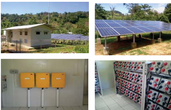
Figure 2. Components of the PV project in Boalemo village
