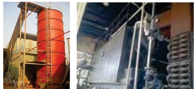
Figure: Biomass boiler feed by wood chips – source: Nam Thai Nguyen - http://ntn.xemweb.net/index.php?mod=article&func=view&id=2569&cid=1713
