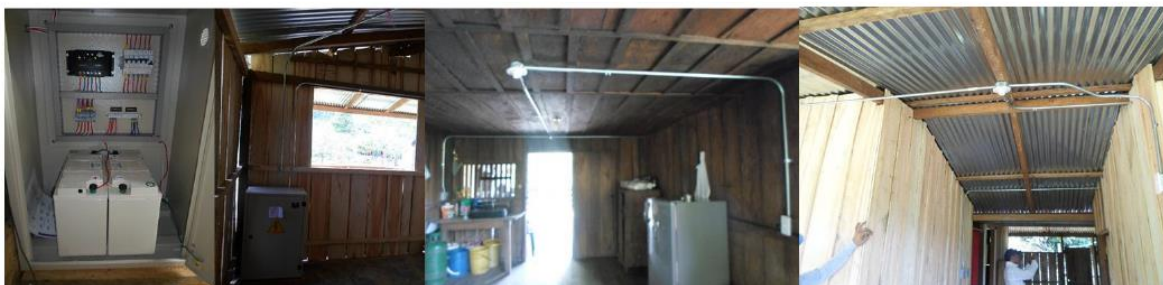
Figure 20 Electricity connections and cabinets.
