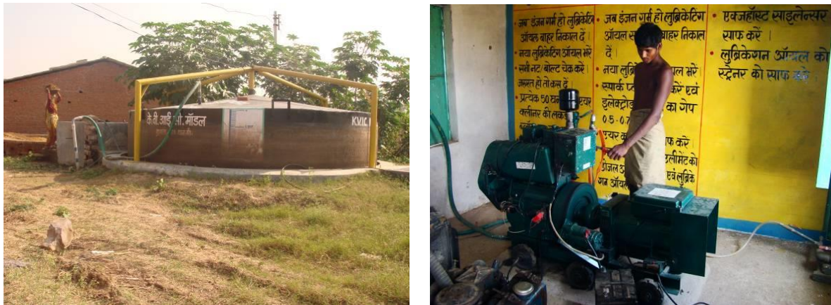
Figure 3. Biogas plant and generator to produce electricity
