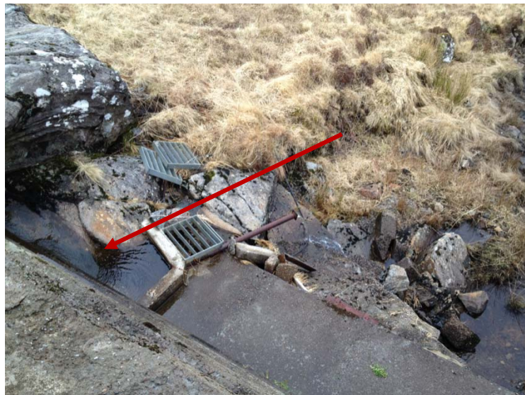
Figure 10: Leakage in the dam 2012
