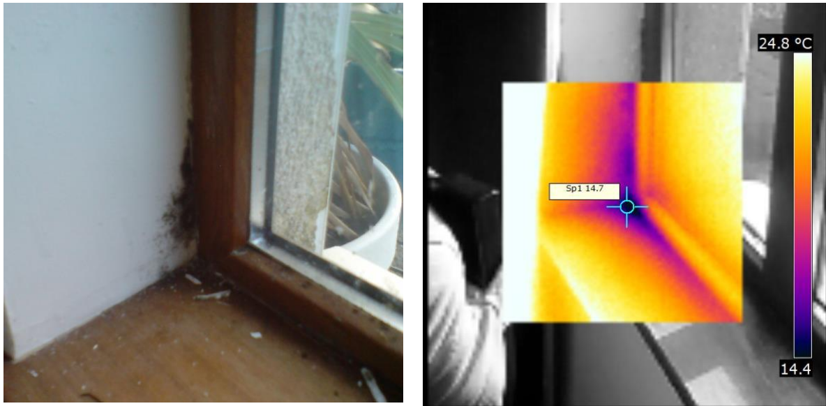
Figure 6.1: Infrared and digital image of the windows. Source: Thermal camera
