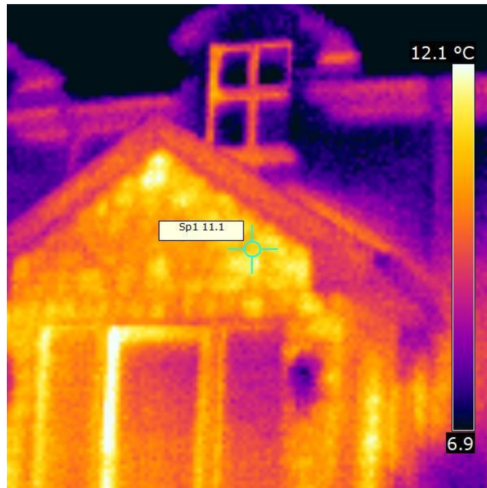
Figure 6.4: Infrared image of the porch. Source: Thermal camera
