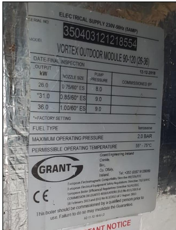
Figure 5.6: Condensing oil boiler name plate Source: Author
